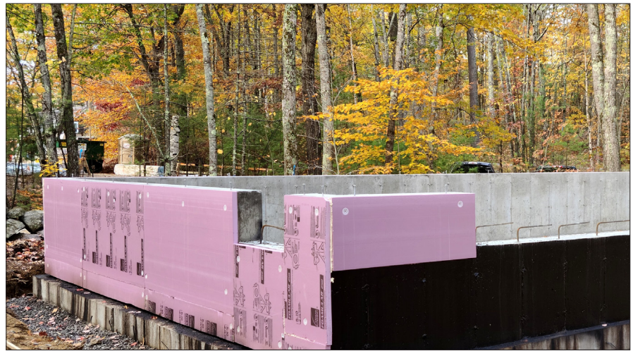
The foundation for the new Kittie and John Wilson Field Operations Center: living quarters for seasonal field biologists and veterinary interns and working and storage space for field equipment and supplies.
